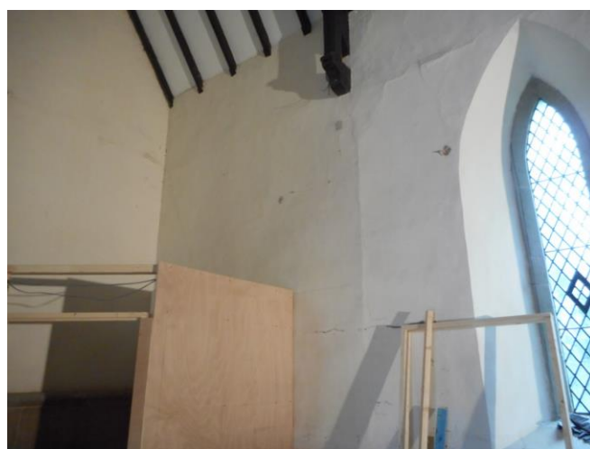
The north-west corner of the chancel, showing extensions to the east and the raising of the roof
