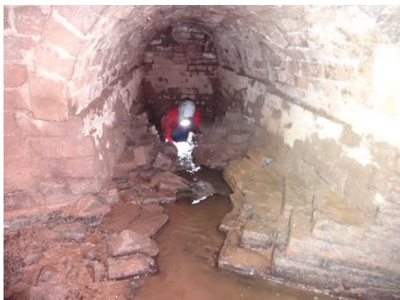
A club member climbs into the upper culvert level at Eardington Upper Forge
